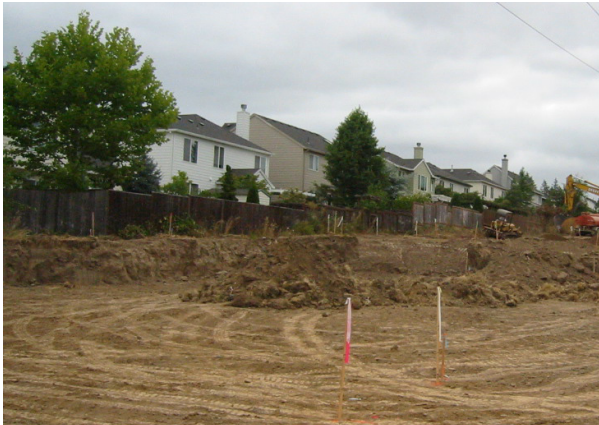
The first phase of work for Kaiser Woods Park included extensive earthwork to create usable spaces on a hillside site, connected by an ADA-accessible trail.
