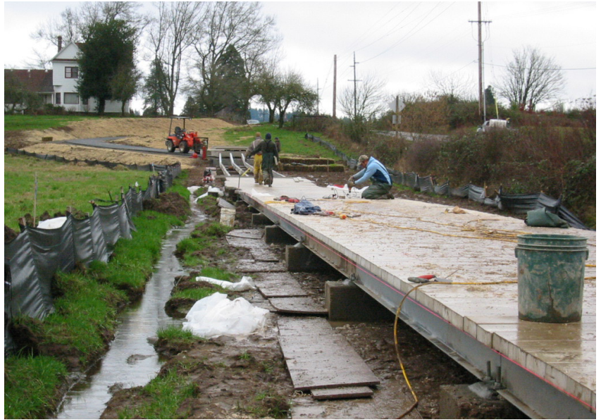
The Stafford Basin Trail included construction of a 250-foot boardwalk across a wetland, turning a perceived obstacle into the highlight of the trail. The boardwalk has a steel frame with recycled plastic decking that will require less maintenance than a traditional wooden boardwalk, but maintains the look and feel of wood.
